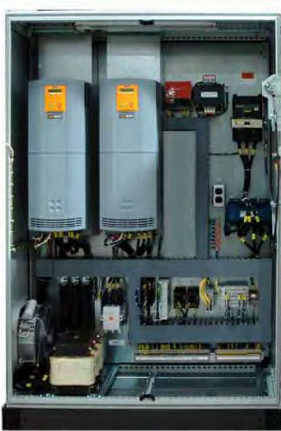
Illustration shows typical panel including AC690+ with AFE and additional system components.
