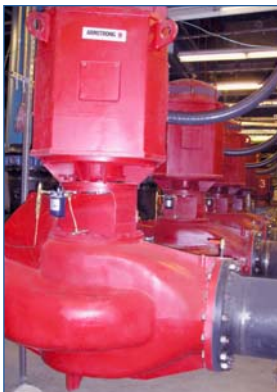
Enwave District Cooling Facility, Toronto, Canada.
