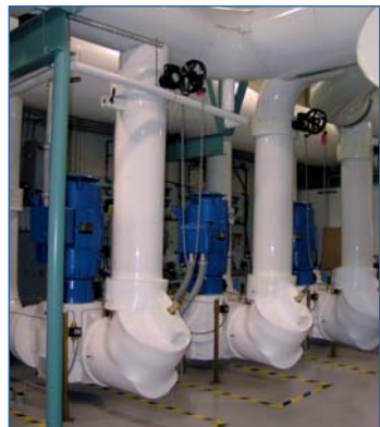
District Cooling Project, Phoenix, U.S.A.
